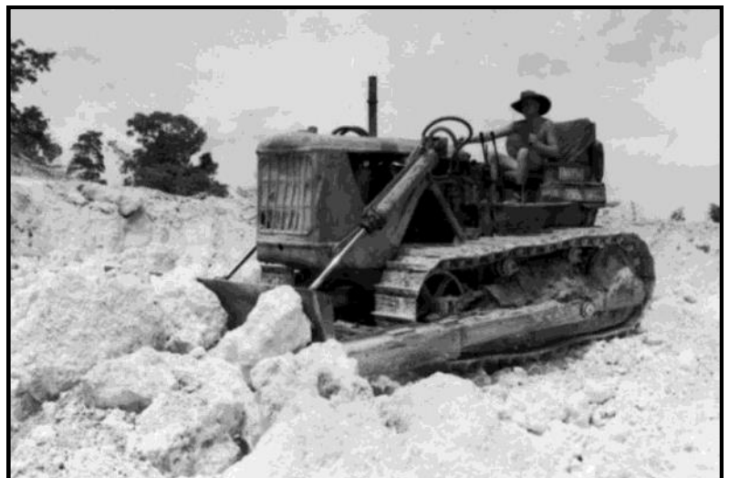
A No. 5 Airfield Construction Squadron bulldozer working in a coral quarry at Noemfoor Island during Dec. 1944.
